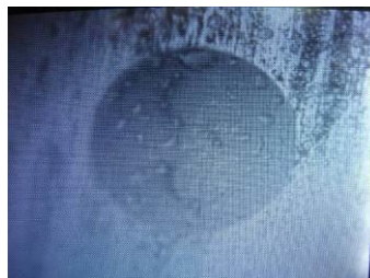
Dirty: Cleaning required
