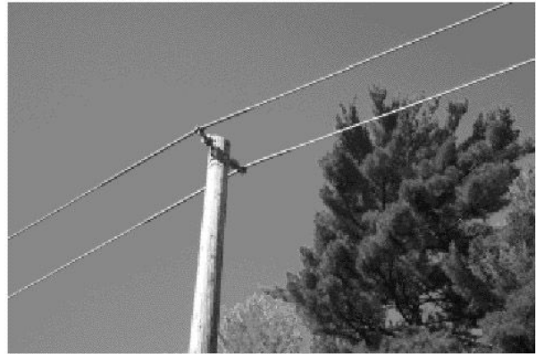
View of a typical Clam Lake ELF antenna
