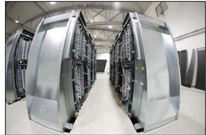
IBM cloud computing data center (1,994 of servers)
